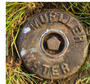
This is what your water service valve looks like that you'll need to mark.
